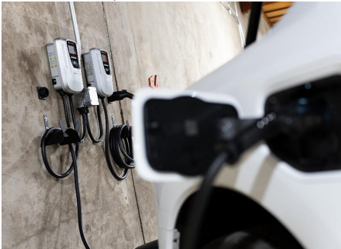
These EV chargers at the Cowlitz Indian Tribe Transportation Center are powered by solar panels and funded in part by the CCA.
