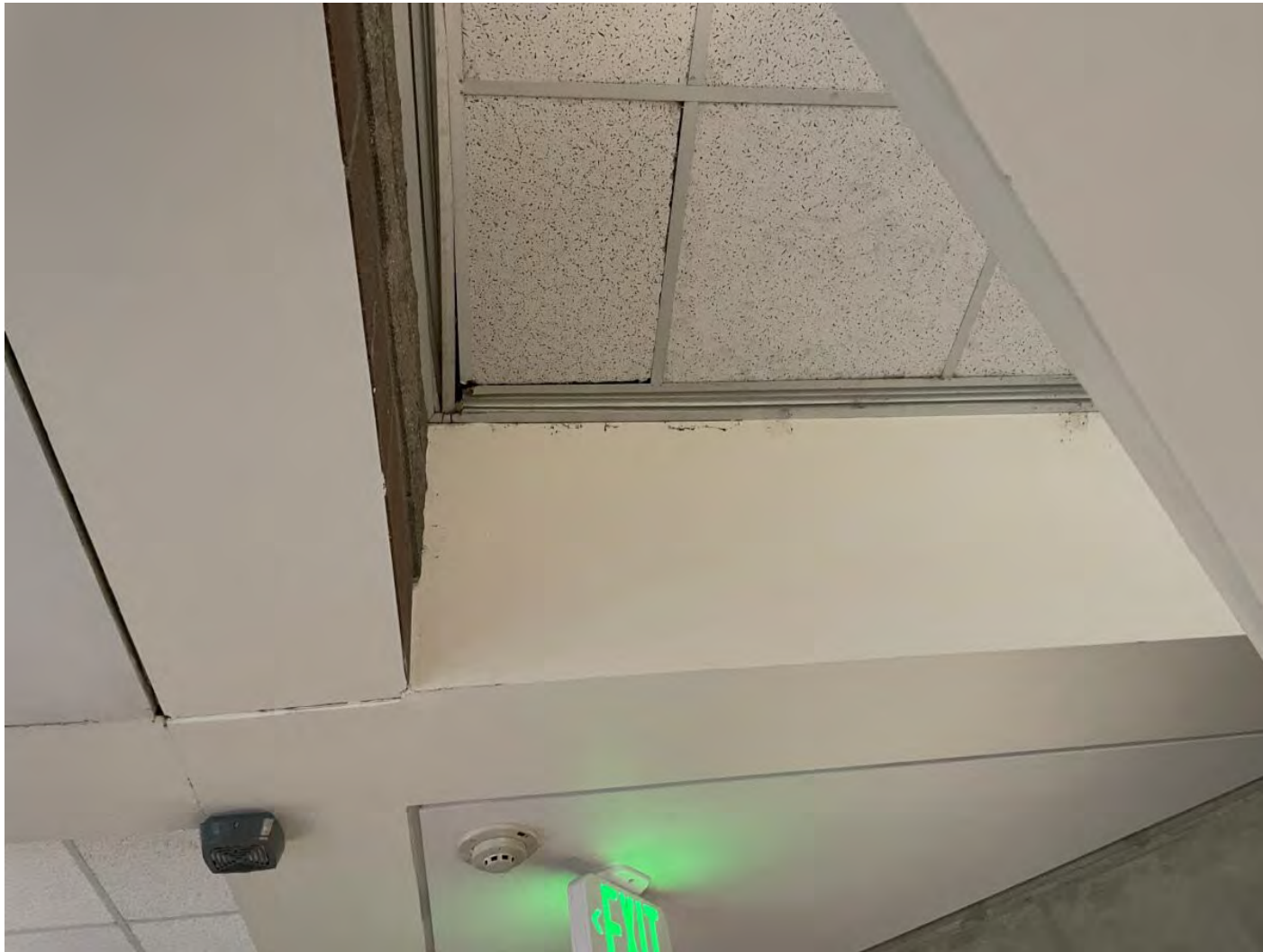
T-Bar and wall connection concerns
