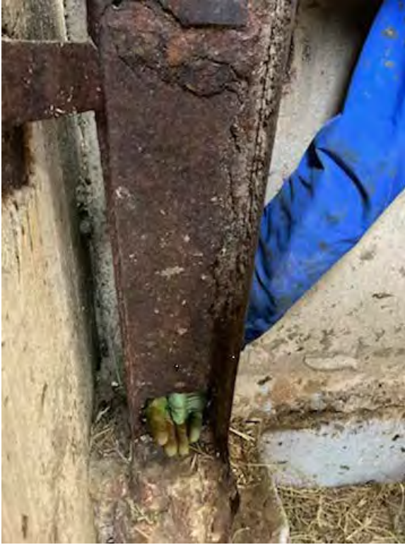
Figure 2 – corroded steel column in Building 402A pens
