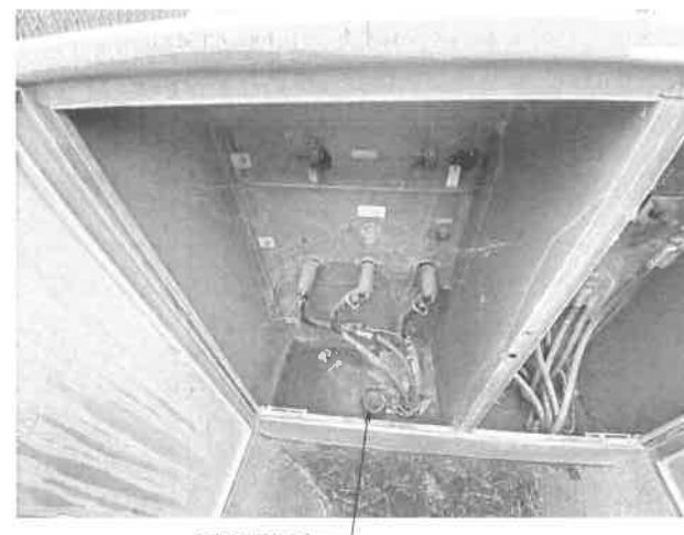
1 MORRISON XFMR #14 INTERIOR - EXISTING N.T.S.
