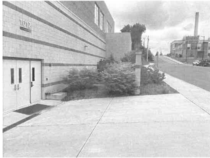
1 REC CENTER XFMR #54 LOOKING WEST - EXISTING N.T.S.
