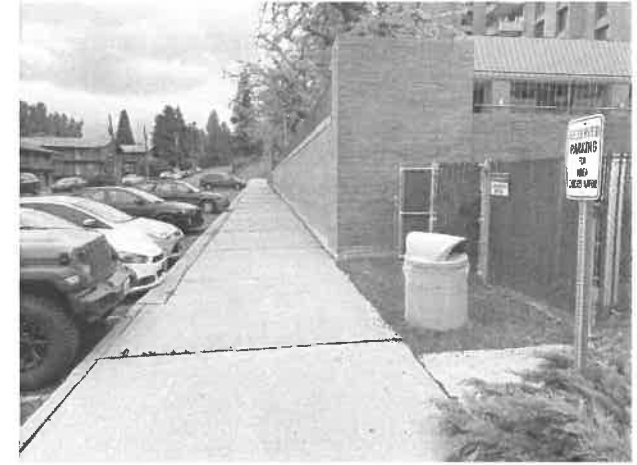
4 STREETER XFMR #15 LOOKING NORTH - EXISTING N.T.S.
