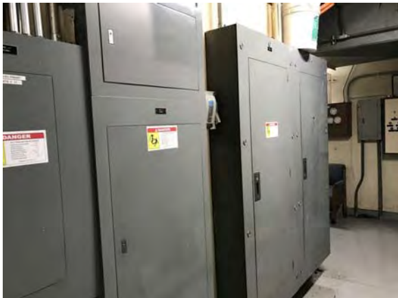
001035e 2/28/2019 Local panelboards Room 130
