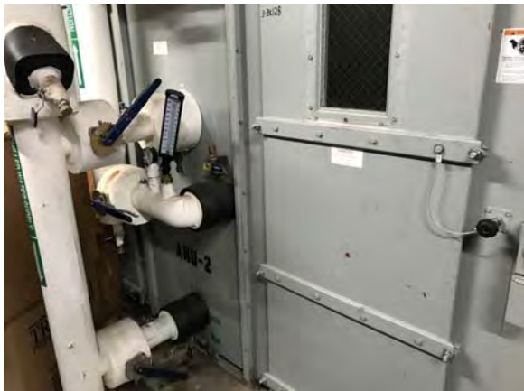
Air handling unit AHU-2 Room 130
