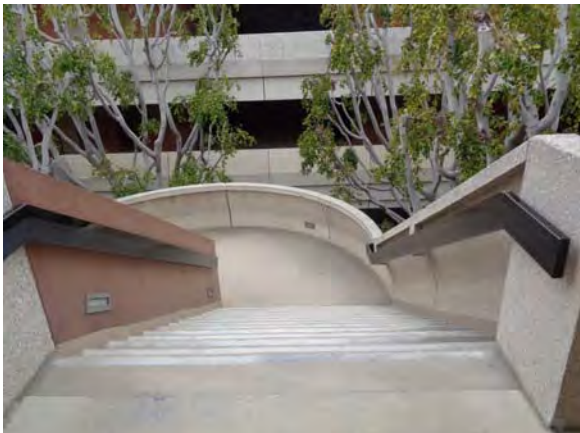
001036a 2/28/2019 Open stairwell with nongraspable handrails Third floor, stairwell SW302
