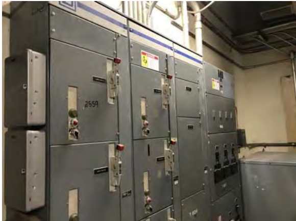
001034e 2/28/2019 Motor control center Room ME0108
