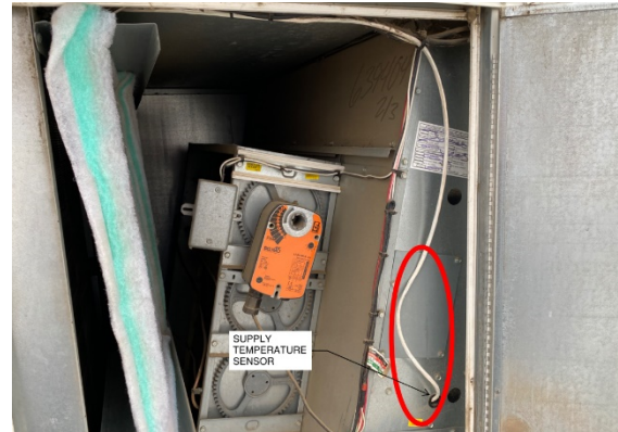
Figure 4 RTU with Bypassed Controls
