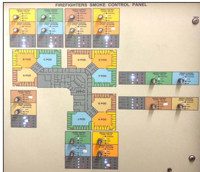
Figure 2 Existing Smoke Controls
