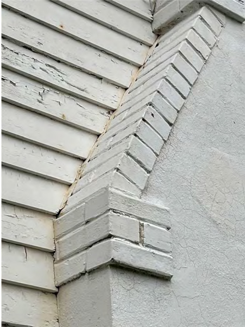
Metal flashing only installed at sloped top of chimney. No caulk at any joints or has failed or missing.
