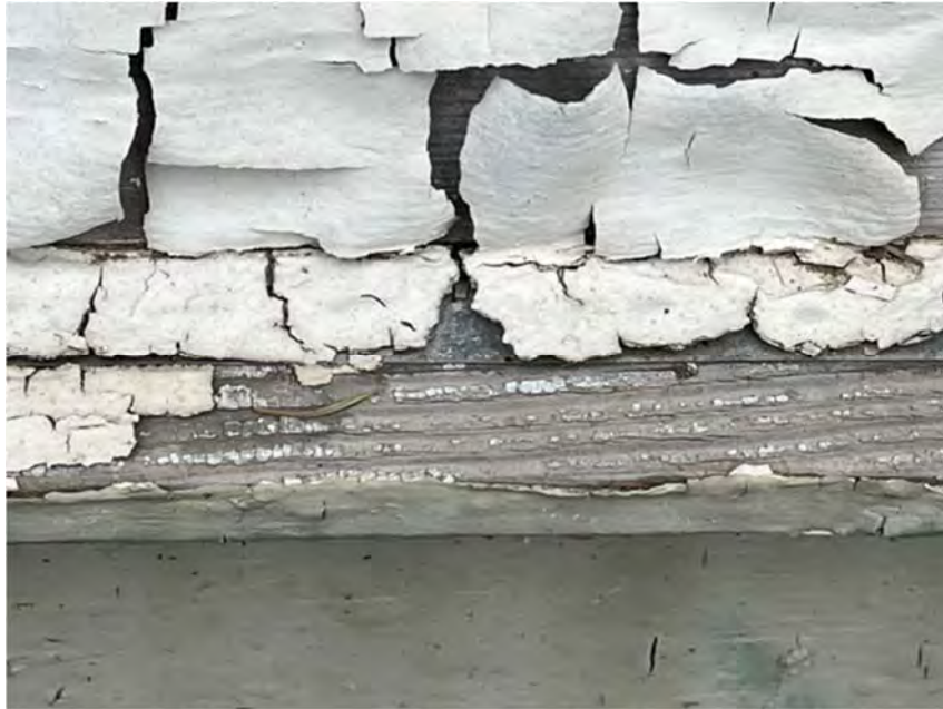
Exterior lap siding with paint finish peeling and cracking off the surfaces, metal flashing didn't extend to protect wood trim at the base of the exterior walls.
