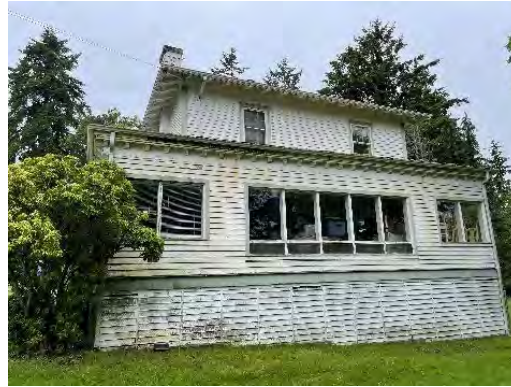
Figure P.4: Gutters and Downspouts
