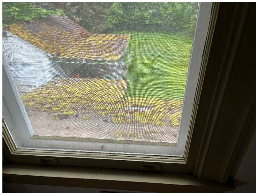
Roofs (viewed through window at upper floor) over existing porch and garage structure are covered with vegetation and appear to be badly deteriorated over the years.
