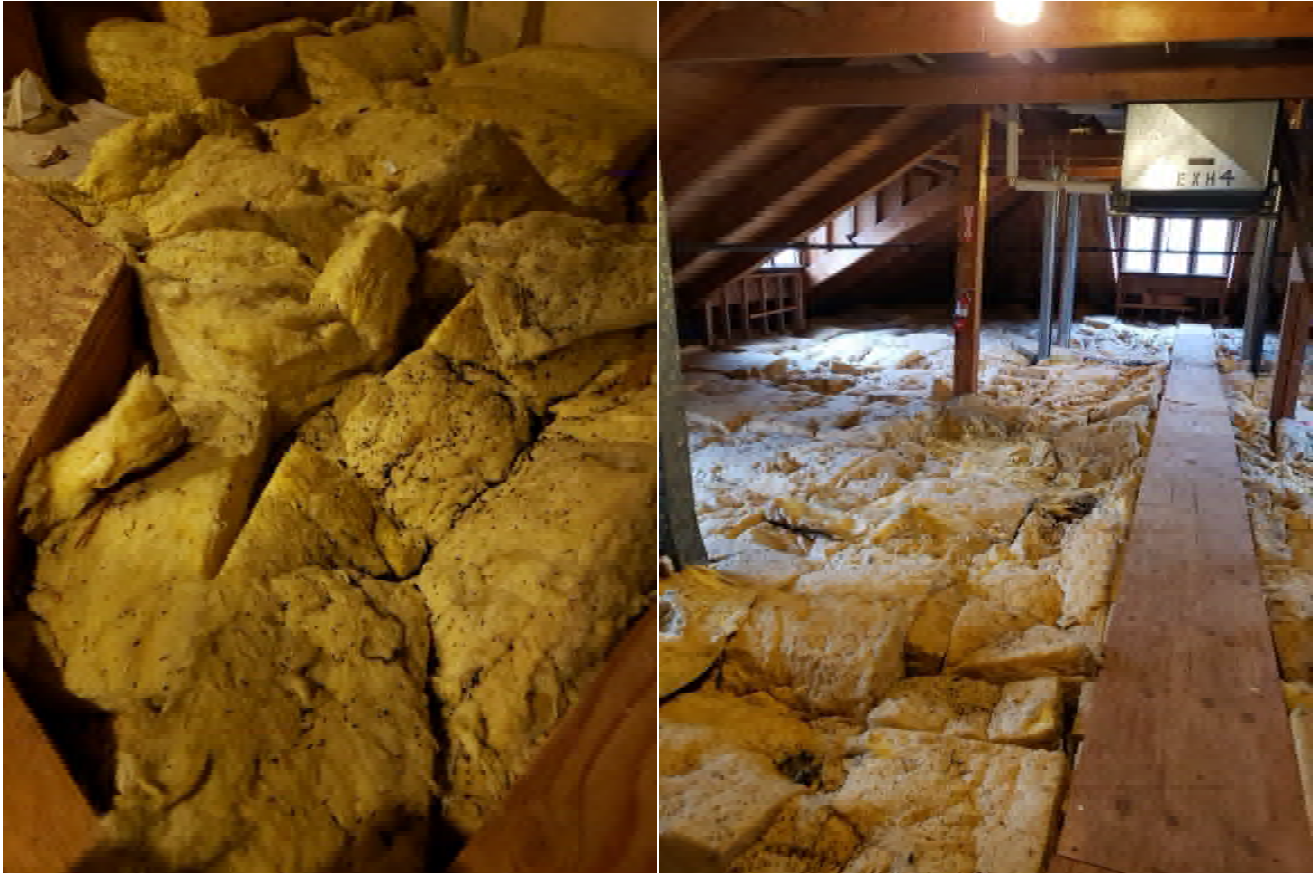
Figure 3. Damaged and bat guano contaminated insulation in attic (left and right).
