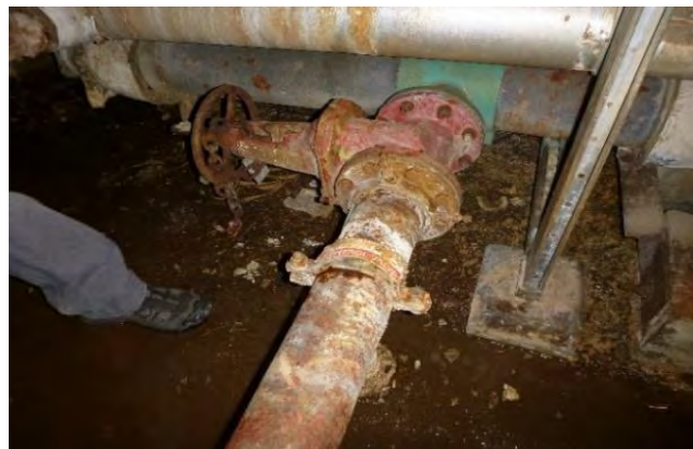
Figure 2: Aged Steam Distribution System
